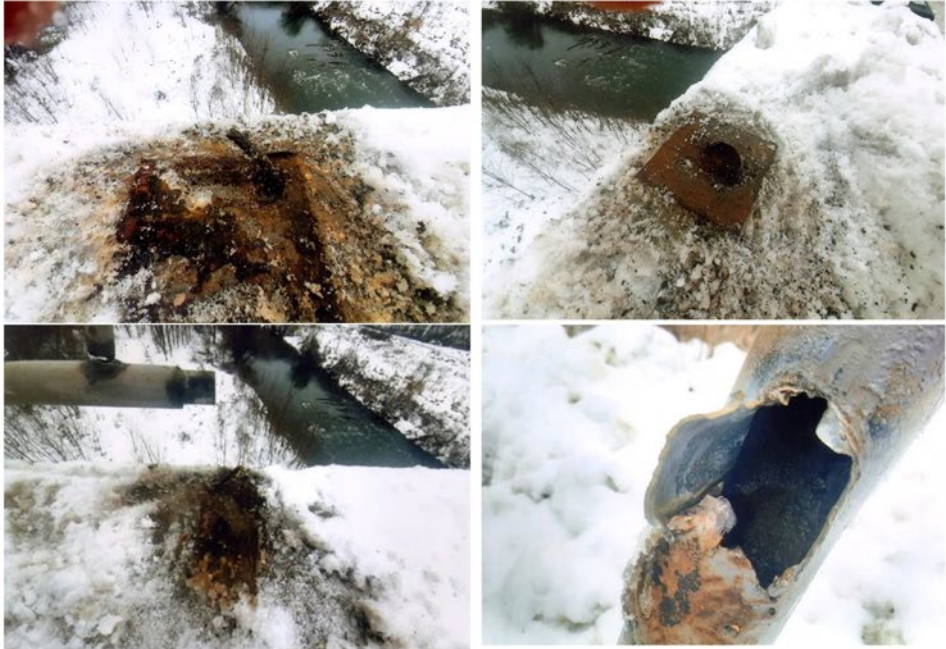
Fig. 2, 3, 4 and 5: The appearance of details corroded, broken poles and the damaged pedestrian guardrail
